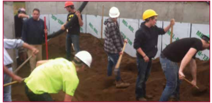
Construction Trades Students Preparing the Basement for Cement on their Project House
